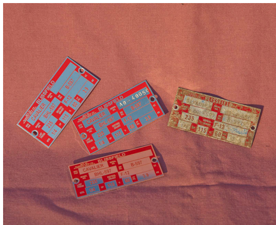
Blissfield Refrigeration Data Plate
